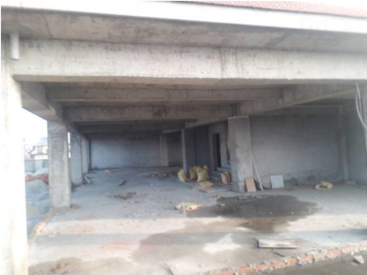
The top roof for our Solar panel :
